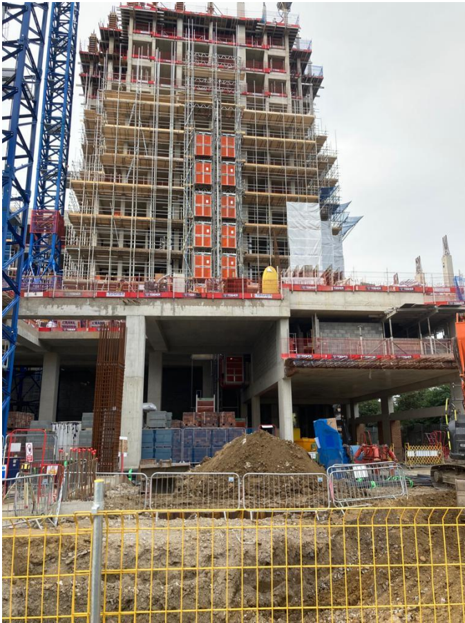
227-255 Ilderton Road under construction showing logistics space in the ground floor podium
